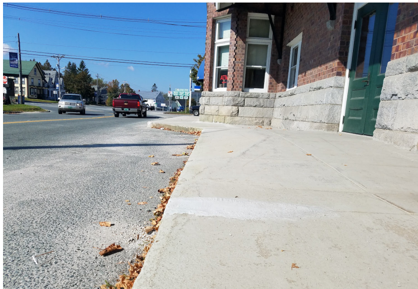
Excessive sloped sidewalk creates hazards during winter or wet conditions.
